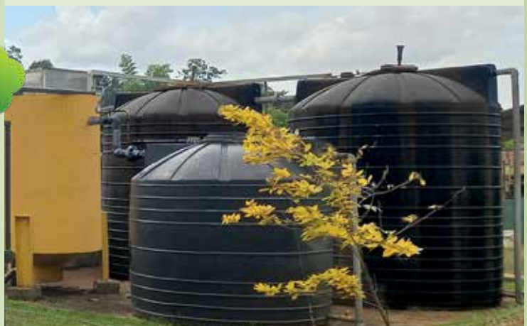
Water treatment plant at Mabima Cylinder filling facility.
